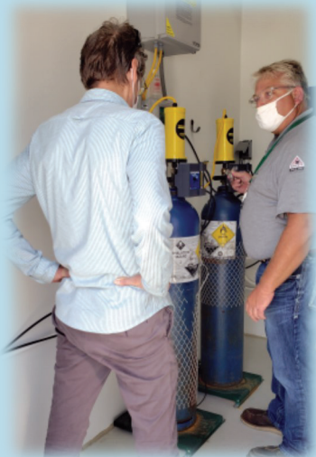
Wayne Guyette details the chlorination process.
